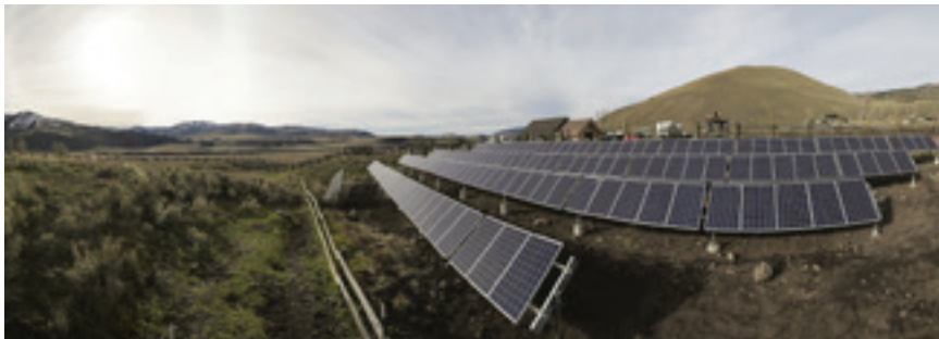
At the Lamar Buffalo Ranch field campus in Yellowstone National Park, 208 reused Toyota Camry Hybrid battery packs (bottom) store energy generated by solar panels (top) in an innovative distributed energy system.
