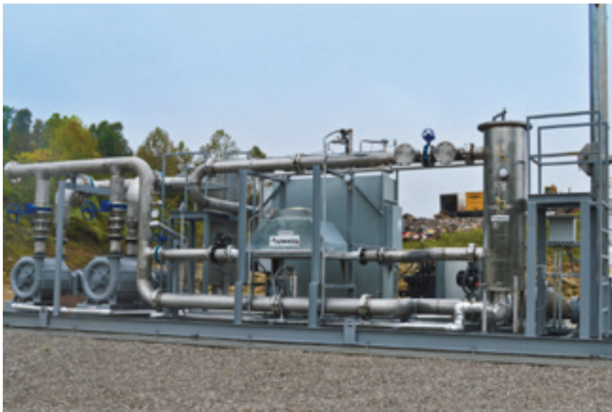
Toyota’s plant in Kentucky (TMMK) teamed up with Waste Services of the Bluegrass to generate power from local landfill waste. The blower/flare skid, shown here, is part of the system that extracts gas from the landfill, conditions it and supplies it as fuel to a generator at TMMK. Toyota estimates the landfill gas will supply enough power each year for the production of 10,000 vehicles.
