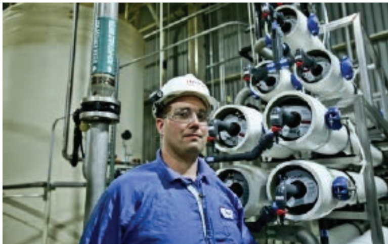
Paul Delor, Environmental Specialist at Toyota Motor Manufacturing, Indiana, stands in front of the plant's reverse osmosis concentrate recovery system. This system is saving the plant 15 million gallons of water per year, or enough water to supply over 100 U.S. households annually.
