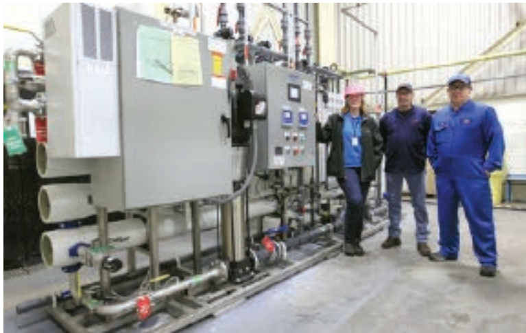
In an effort to reduce water use, Toyota team members Bethany Giordano, Jeff Bacchus and Doug Brinker have been implementing a brackish reverse osmosis system at Toyota’s Georgetown, Kentucky, assembly plant. This system allows the plant to save nearly 17 million gallons of water a year.
