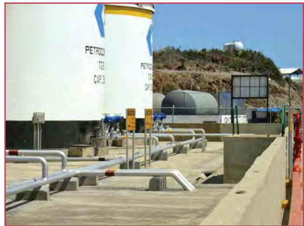
The Baltra fuel handling facility, once an environmental and safety hazard, is now a technologically-advanced facility.
