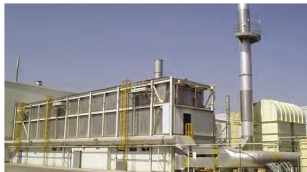
Paint ovens are located on the exterior of the paint shop at TMMBC in order to reduce the cooling needs and related energy usage.
