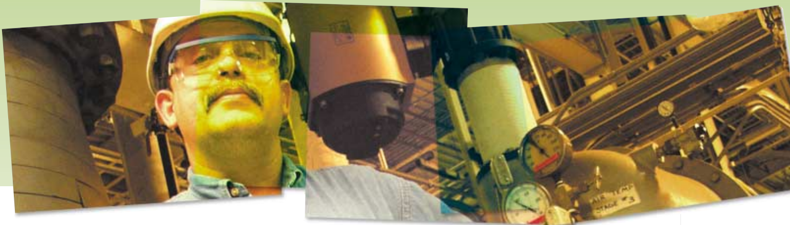
Danny Jackson, Team Leader, inspects an air compressor that is part of Toyota's intensive leak detection program. Reducing the running time of such compressors reduces the company's consumption of energy.
